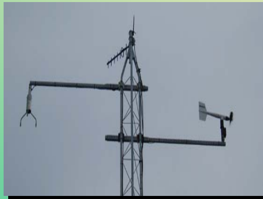
Figure 4. Redundant wind system at Egmont Key
